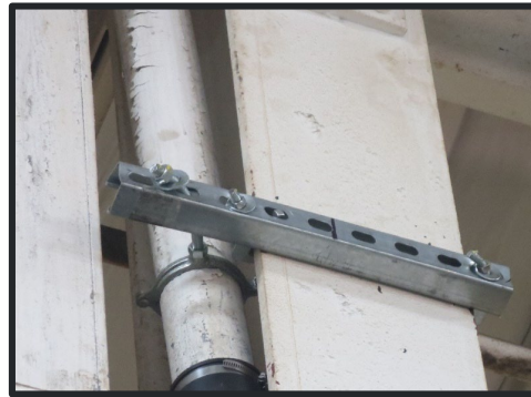
Temporary bracket and bent securing bolts
