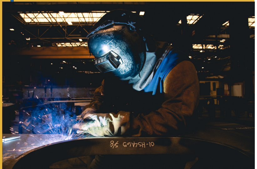
A. Nelson welds an Enterprise (CVN 80) unit in the Steel Production Facility in Hot Shots, June 2021 Photo by Ashley Cowan
