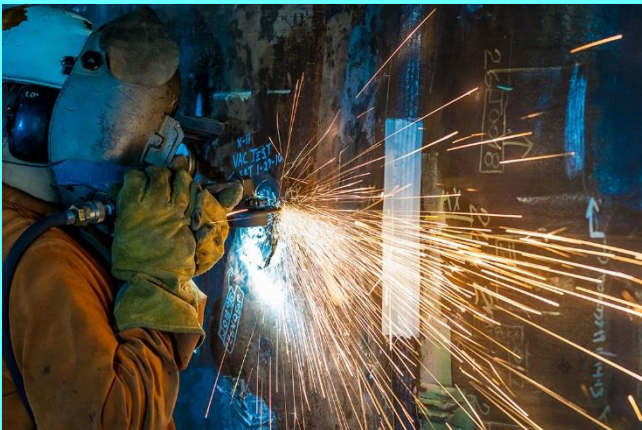
A shipbuilder cleans up welds on the Delaware SSN 791 for magnetic particle inspection. Photo by Chris Oxley.
