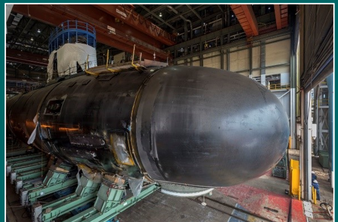
Construction on the submarine Washington (SSN 787) progresses in the Modular Outfitting Facility. Photo by Chris Oxley
