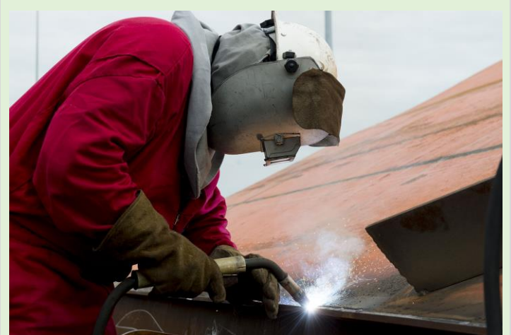
Welder Bobby Vaughn works on the aircraft carrier USS JOHN F. KENNEDY (CVN 79) Photo by Ricky Thompson
