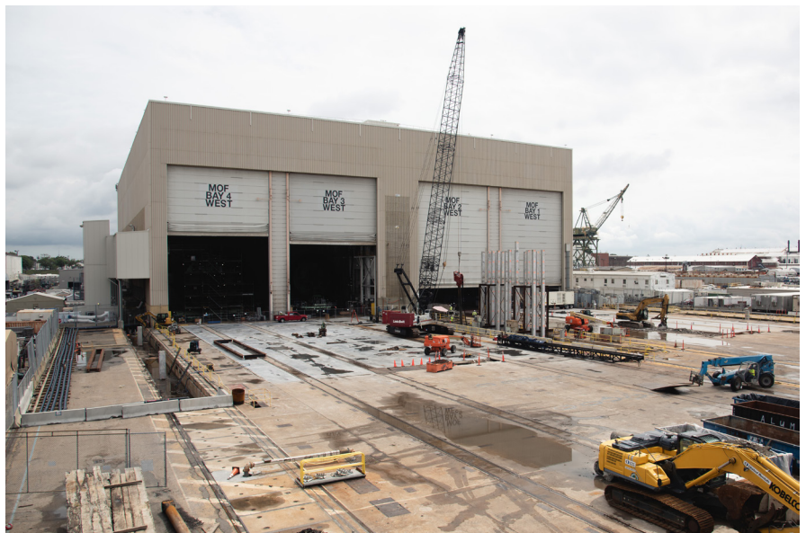
Work is underway for a 200-foot extension to the Modular Outfitting Facility (MOF). Photo by Matt Hildreth
