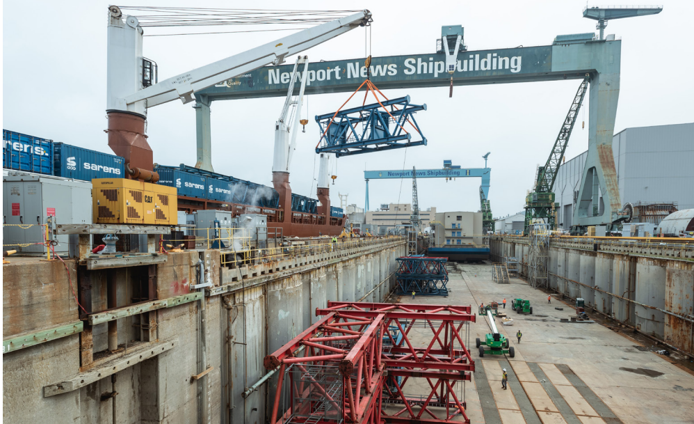
Lifting equipment that will be used to help disassemble the crane is lowered into a dry dock. Photo by Matt Hildreth
