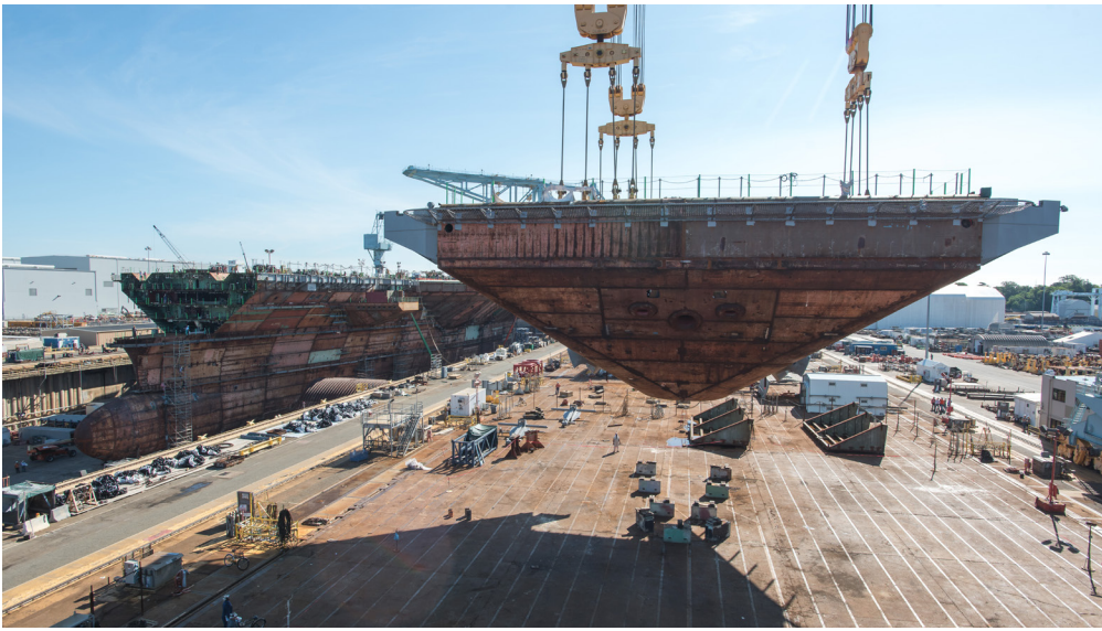
The superlift that completed Kennedy's flight deck weighed 780 tons. Photo by Ashley Cowan
