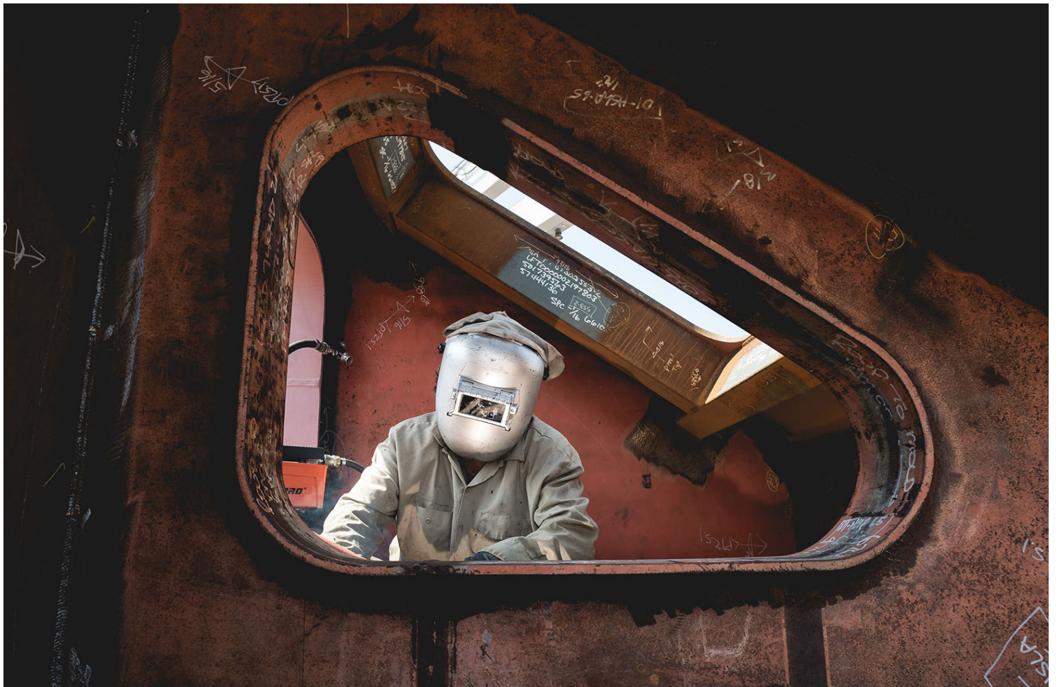
Check out August Hot Shots. In the photo above, Tommy Morse is framed by a coaming on a John F. Kennedy (CVN 79) unit as he performs welding operations. Photo by Matt Hildreth
