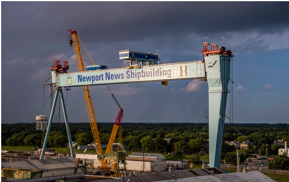
The girders of Newport News Shipbuilding's new 315-metric-ton Goliath gantry crane were lifted into place Aug. 4-5. Photo by John Whalen
