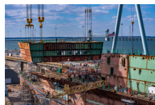
Cover Photo: An 806-metric ton superlift for John F. Kennedy (CVN 79) is hoisted into place. Photo by John Whalen
