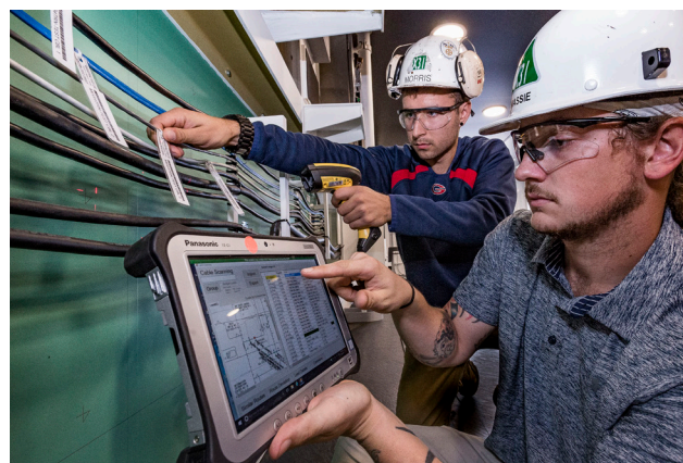
From left, Chad Morris (X31) and Samuel Massie (X31) use KP-3 technology to map cables. Photo by John Whalen
