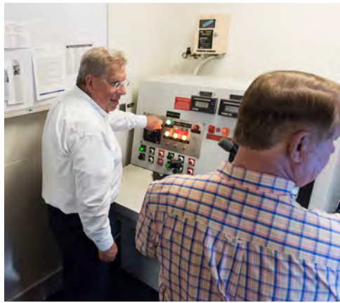
Matt Mulherin waits for a signal from Master Shipbuilder and Power Plant Operator Ralph Gilley prior to sounding the shipyard whistle at 3:30 p.m. June 30. Photo by Ashley Major
