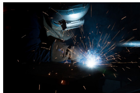
Brandon Sandley throwing sparking in the Modular Outfitting Facility (MOF). Photo by Matt Hildreth
