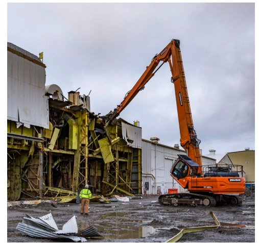
Work is underway to demolish Newport News Shipbuilding’s full-scale propulsion plant mock-up. Photo by John Whalen
