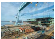
Cover photo: A 704-metric ton unit is lifted into Dry Dock 12 during John F. Kennedy (CVN 79) construction. Photo by Chris Oxley
