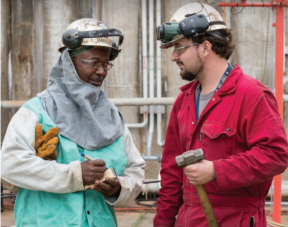
Welder Gerald Barnes (X18), left, and Fitter John Miller (X11) work together to complete a job for CVN 79. Photo by John Whalen
