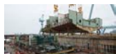
Cover Photo: On April 1, shipbuilders placed the 21st superlift for John F. Kennedy (CVN 79) into Dry Dock 12. Photo by John Whalen
